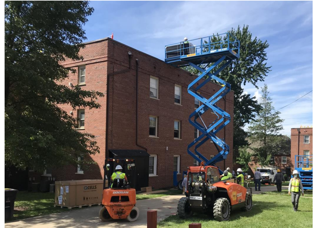
Solar installation at Fairfax Village II
